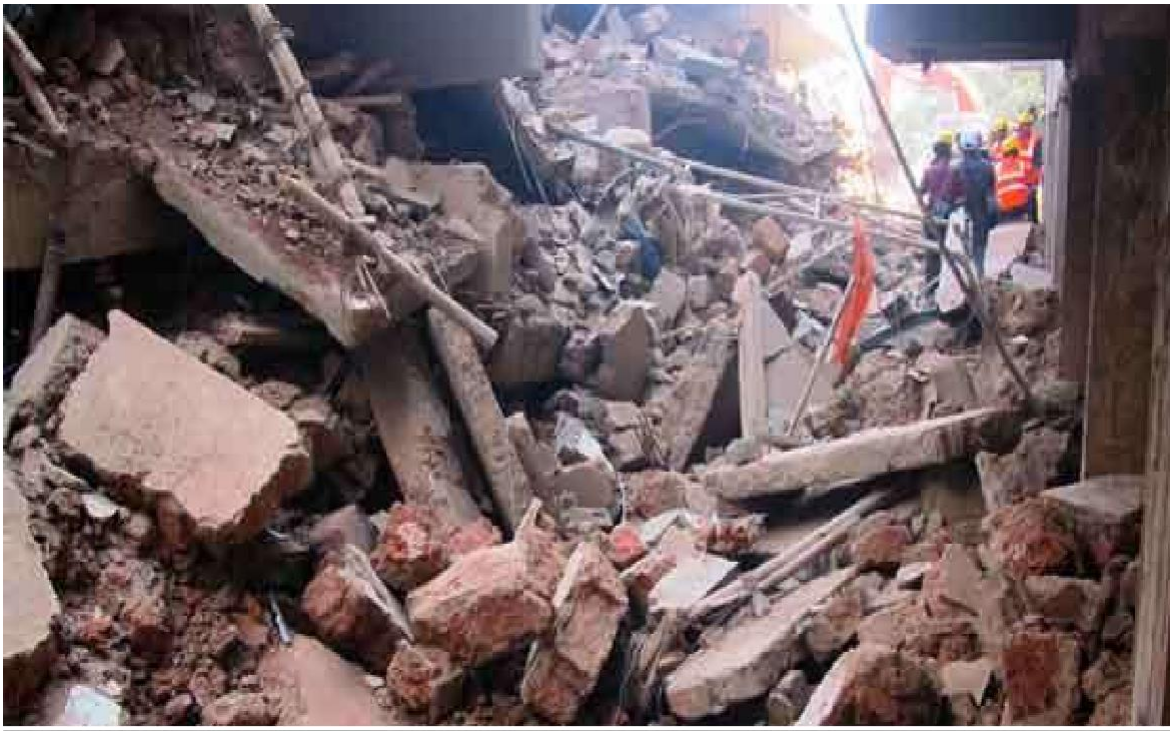
Fig 2: Canacona building after the collapse
