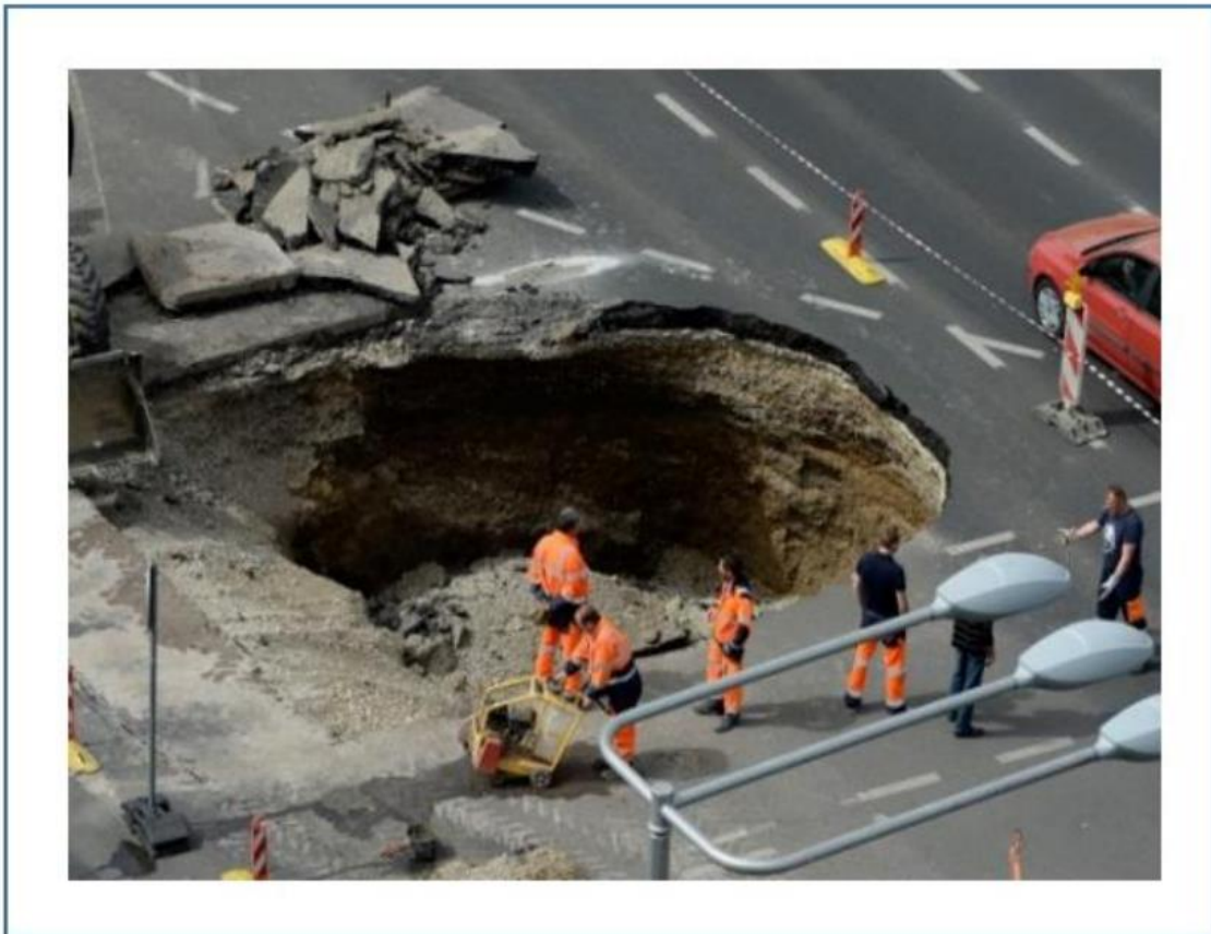
Figure 4.7: Fault undetected in time – indirect damage [izvor: Vodoopskrba i Odvodnja].
