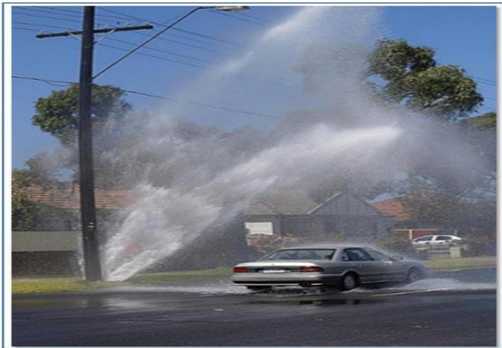
Figure 4.6: Breakage of the water supply pipeline [source: Vodoopskrba i Odvodnja].
