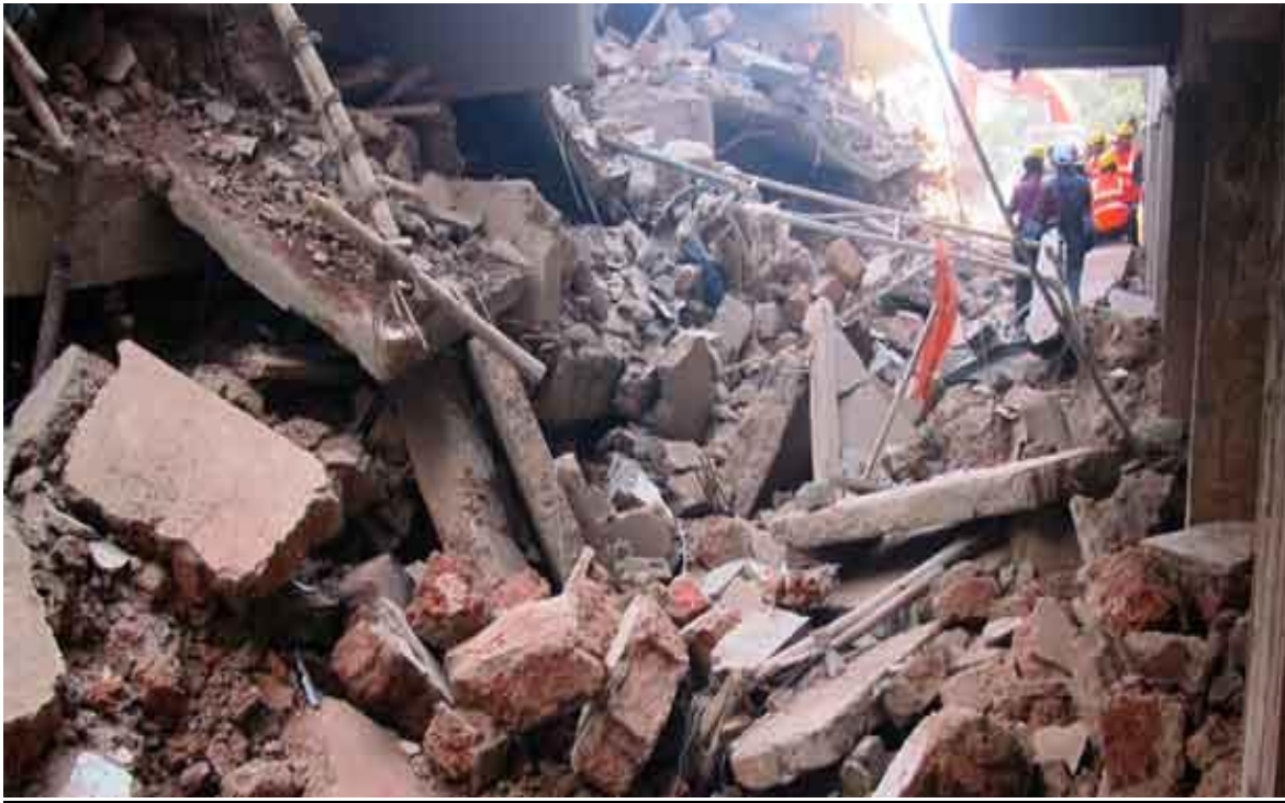
Fig 2: Canacona building after the collapse
